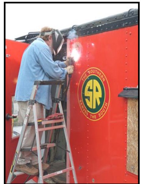
Jim Hopkins welding up some of the holes in the side of the caboose.
