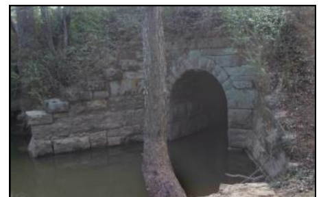
Stone culvert under the old Southern Railway line near Piedmont, S.C., believed to have been built in the 1850's. Photo by: Jim Hopkins ©2014
