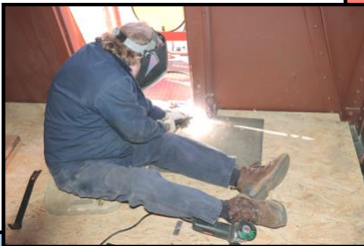
New door threshold being fit and welded in place by Jim Hopkins. Nice industrial look for the caboose.
