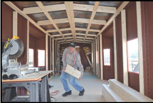
Bruce Gathman carrying another heavy load of 12x4s. Interior framing of walls and ceiling complete.
