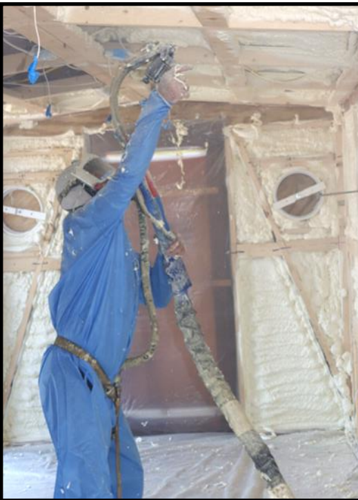
Foam Insulation Co. applying the closed cell foam to the interior of the caboose.
