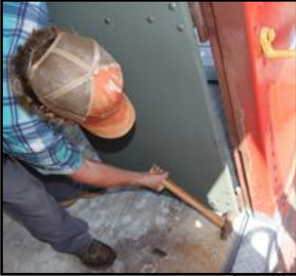
↓ Jim Hopkins drives final hinge bolt home in the new metal caboose end doors.
