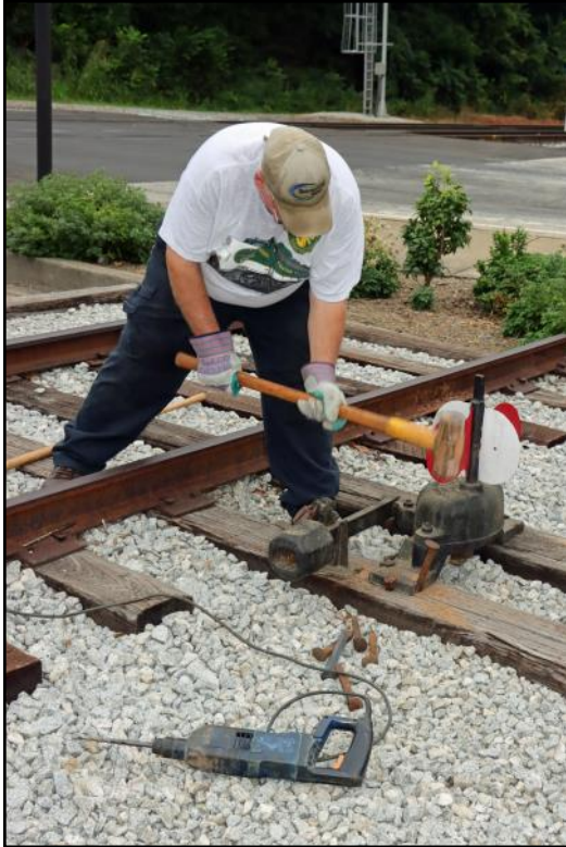
↑ Bob Klempner gives his best imitation of a Gandy Dancer driving spikes in the newly installed low level switch stand at the caboose.
