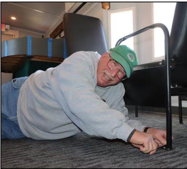
Bob Klempner laying down on the job again. He is shown bolting the newly refurbished caboose chairs to the floor.
