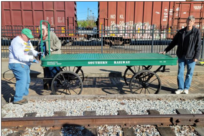
Work crew is placing the first of two restored baggage wagons at the museum. Second will be placed by the museum exit on the trackside of the building.
